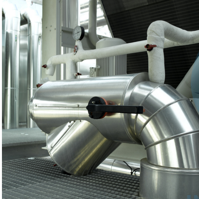
Air conditioning application
